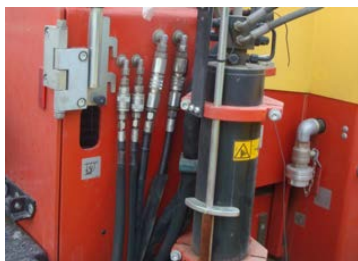
Fig. Hose connect to conveyor motor
